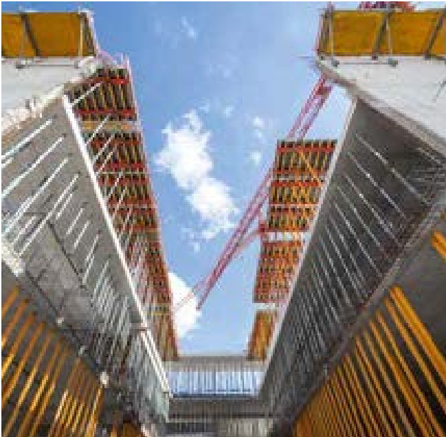
The Folding Platform FB 180 together with the MAXIMO Wall Formwork ensured that the strict tempo specifications could be met.
