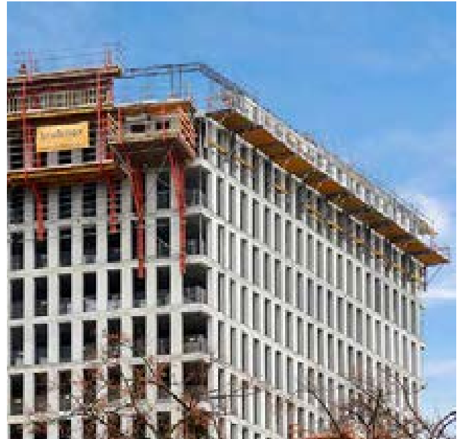
On-site assembly of the Folding Platform FB 180 proved to be quick and straightforward as it was delivered to the construction site in a pre-assembled state.
